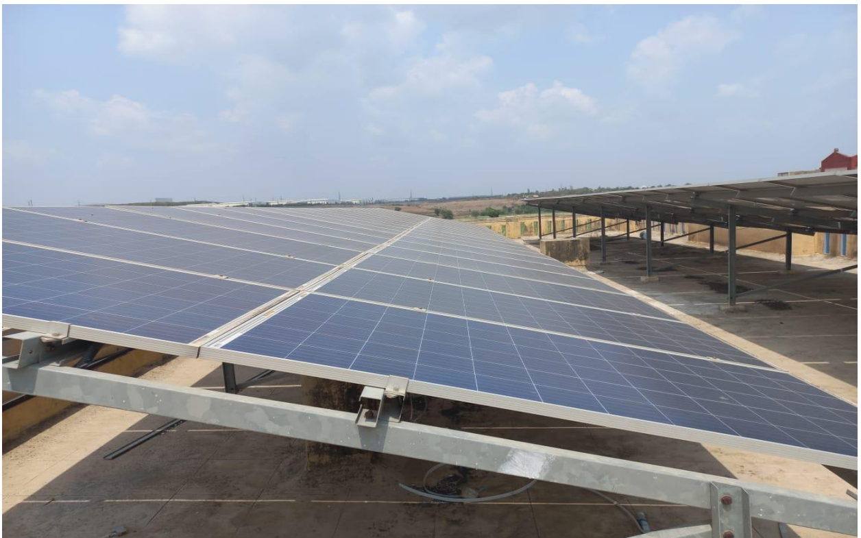
Photo-5: 221 kW solar roof top on Siddhant School building roof.
