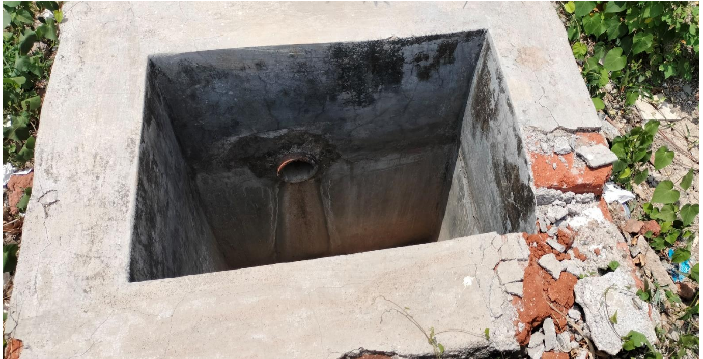
Photo-6: View rain water collection from building
