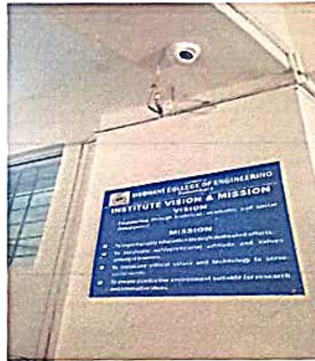
Photo: CCTV camera in corridor outside classroom
